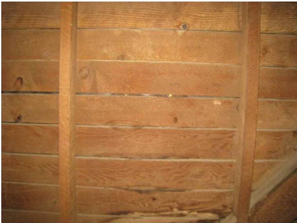
Figure 29 - West wall of south tower (north tower similar). Wall framed w/2x4s @ 32" OC and 1x6 board siding. Exterior finish is diamond-shaped shingles of terne-metal with no vapor barrier apparent. Daylight shows between planks penetrating voids between shingles. The attic of Old Main is un-insulated including the central roof, the perimeter Mansard and tower roof and walls.
