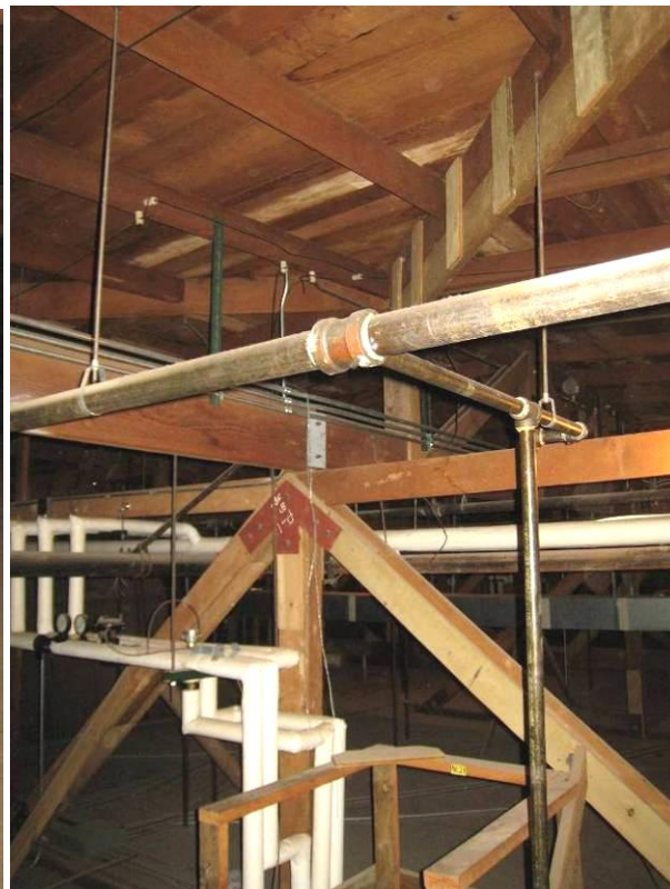
Figure 19 - Fire sprinkler and HVAC piping @ attic of central roof section; note diagonal propped hip rafter for roof pitch, with additional wood stiffener scabbed on beneath.
