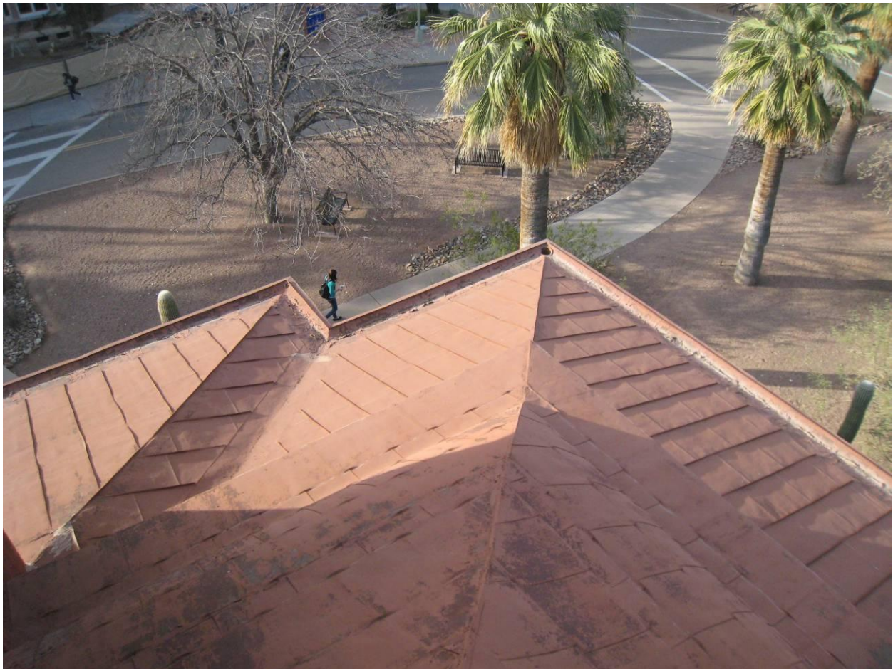
Figure 11 - Hip seam at SW corner of curved Mansard roof, with standing seam at porch roof below & beyond. Gutters at porch eaves routinely become clogged with accumulated dust & debris turned to solid adobe.
