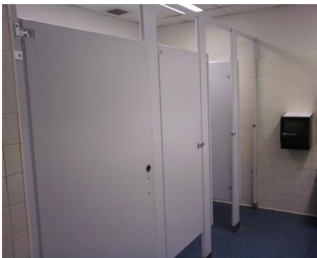
Figure 62 – 2 nd . Floor Women’s restroom has four stalls but only 3 toilet fixtures, the fourth stall being modified to provide a wider detail for handicapped access.
