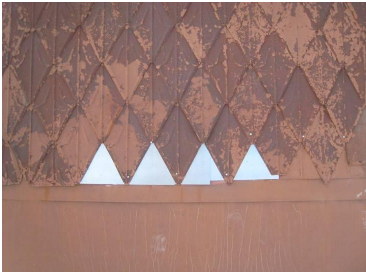
Figure 16 - Details of pressed/stamped terne-metal shingles original to building (1891); Arizona’s oldest roofing. Provisional repairs made w/galvanized sheet metal at north face of south tower (hence in shade).
