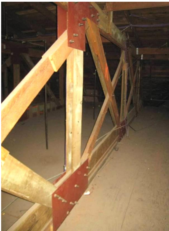
Figure 18 - Original X-braced wood trusses reinforced with steel gusset plates and through-bolts ca.1987. The attic space is well-maintained and organized.
