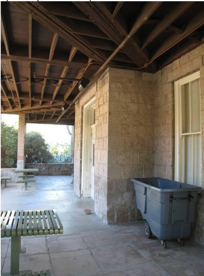
Figure 32- Porch floor structure; decking has deteriorated and joists are rotted.
