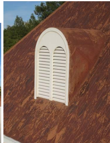
Figure 5 - Rusted sheet metal roofing at ventilation dormer.
