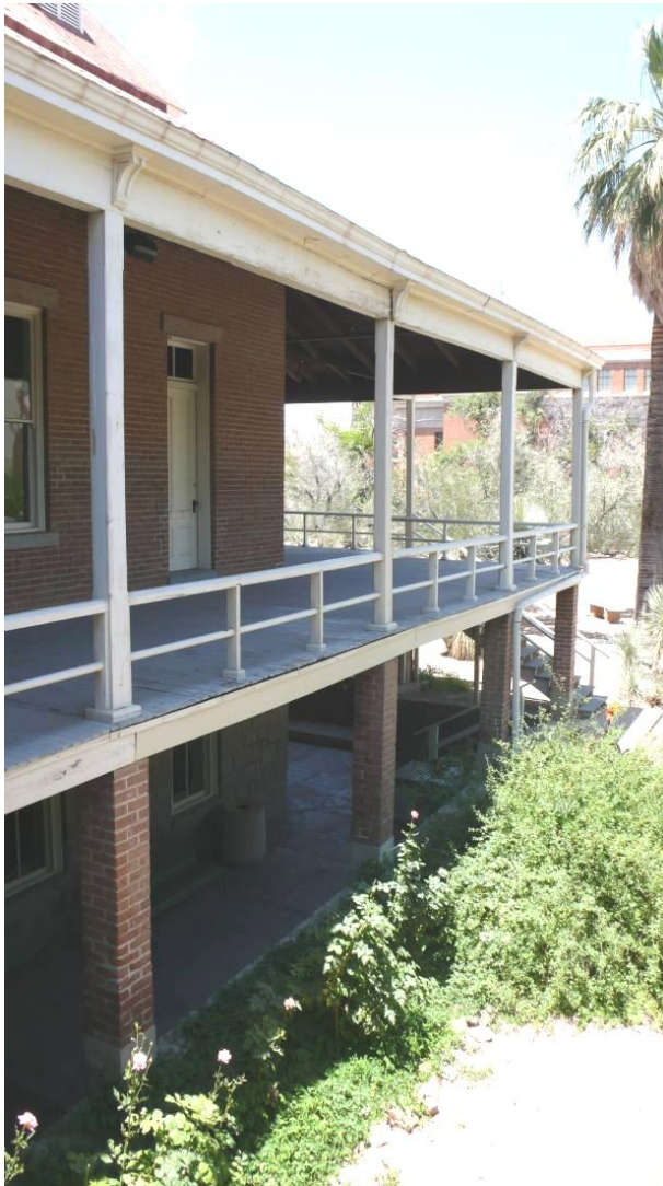
Figure 38 - North east porch from pier #8 to pier #11 note differential settlements at pier #9, as indicated by deflection in eave line.
