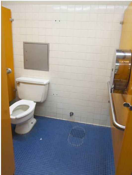
Figure 72 – 2 nd . Floor Men's restroom ADA water closet; re-patching in the tile, after the removal of next toilet to accommodate ADA guidelines.
