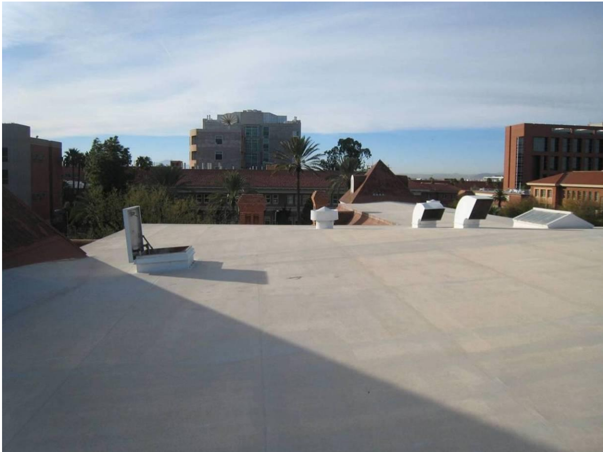
Figure 6 - Central area recently re-roofed with membrane roofing. This originally was roofed with standing-seam metal in a shallow hipped configuration, as seen in the historic photo on following page.
