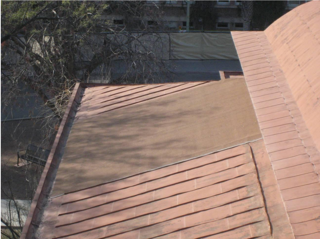
Figure 17- SE wing of porch with deteriorated standing seam metal, a portion of which has been replaced with patch of asphalt roll-roofing with brown mineral cap. Note shallowness of perimeter gutter, which is ineffective.
