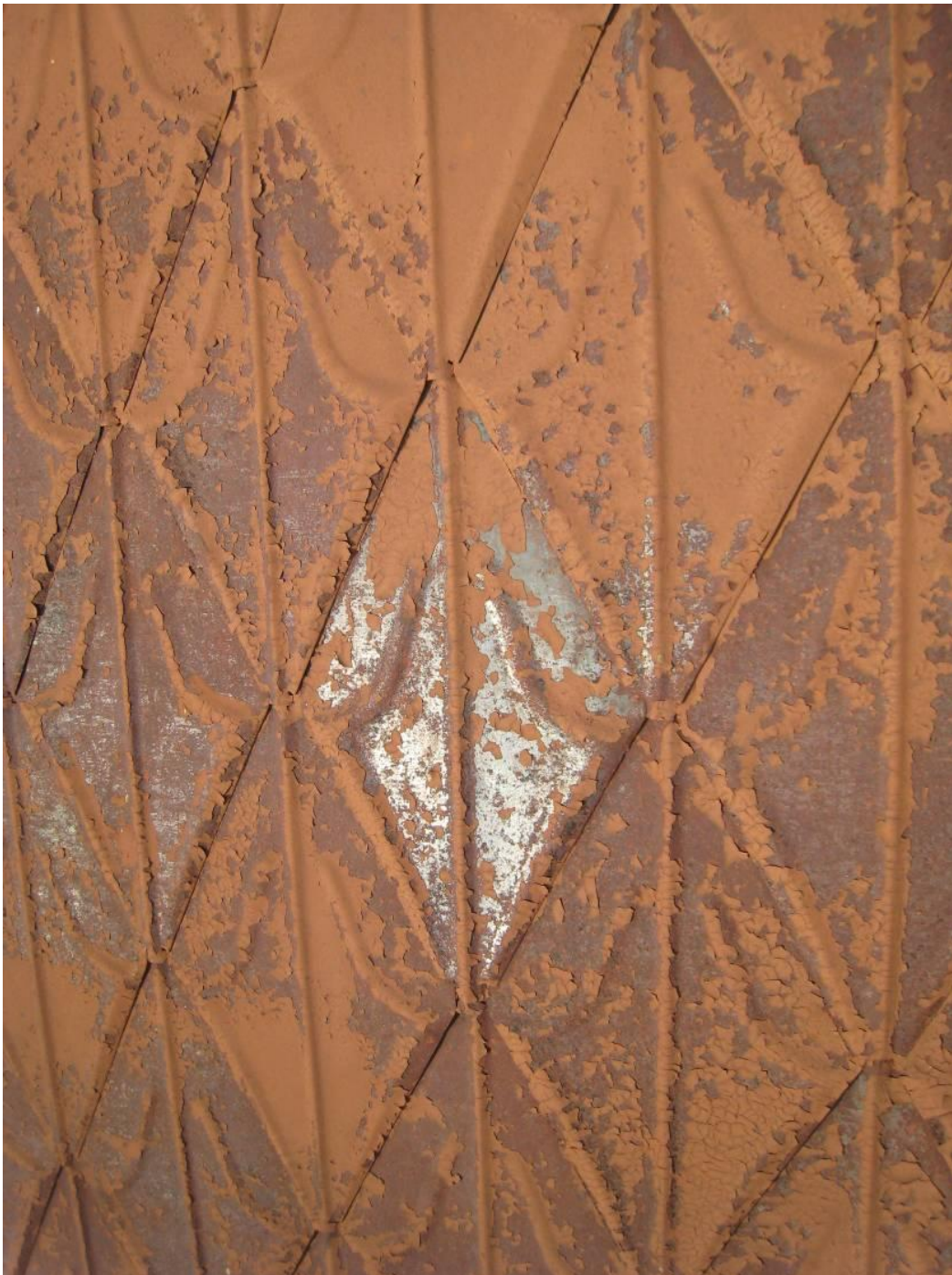
Figure 10 - Pressed terne-metal fish scale shingles used at 4 tower roofs and as wall siding at north & south towers. Severe deterioration is evident. Paint disguised deterioration and prolonged life.
