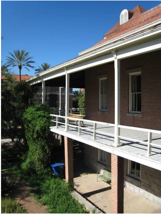
Figure 35 – Pier #48 jack-knifing outward, out of plumb.
