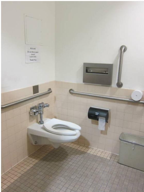
Figure 70 – 1 st . Floor Men's restroom, showing E/O wall mounted toilet and ADA compliance installations.
