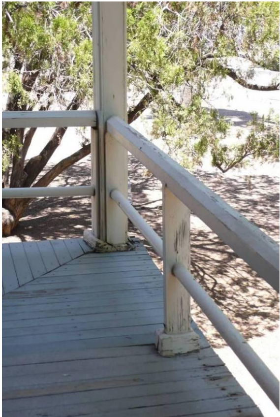
Figure 36 - Deteriorated deck & base at post # 11.
