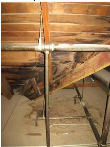
Figure 23 - Roof leaks at valleys and hips have damaged wood framing over time.
