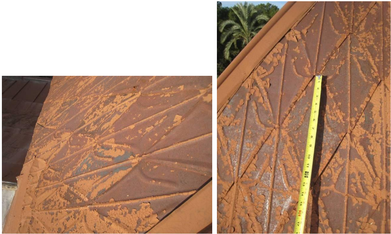
Figure 15 - Traces of lead & tin terne coating remain on a few tiles. Diamond shaped tiles measure 7½”w x 13”h.
