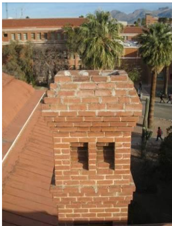
Figure 3 - Chimney requires re-pointing w/ compatible lime mortar and lateral reinforcing.
