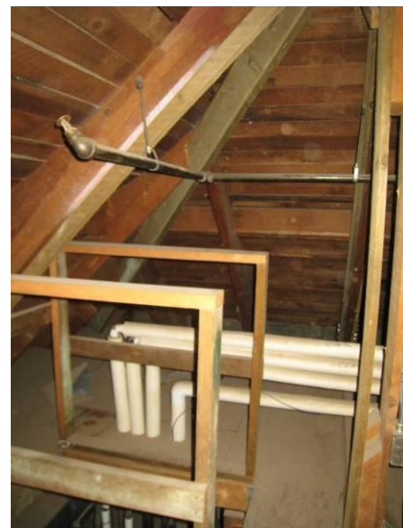
Figure 24 - Hip rafter adjacent replaced w/pressure treated 2x6 (note green tint)
