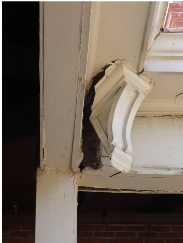
Figure 37 - Deteriorated wood & sheet metal bracket at post #7.
