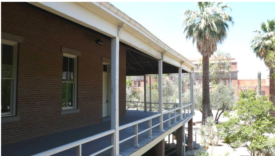
Figure 31 - Perimeter beam at post #9 (second from left) shows deterioration & settlement; this may be due to foundation settlement rather than failure of the beam itself.
