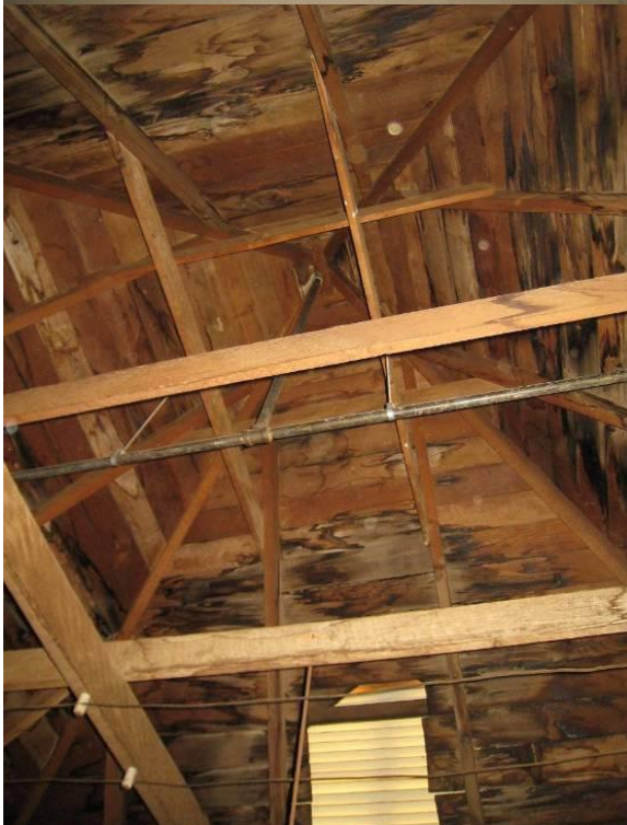
Figure 27 - Interior of south tower pyramid; extensive leaking is evident. Roofing must be replaced as well as 1x6 wood deck affected by moisture. At the towers, approximately 50% of decking appears moisture-damaged. At time of re-roofing, plywood or OSB sheathing should be installed above 1x6 decking, to create a diaphragm for improved lateral stiffness.
