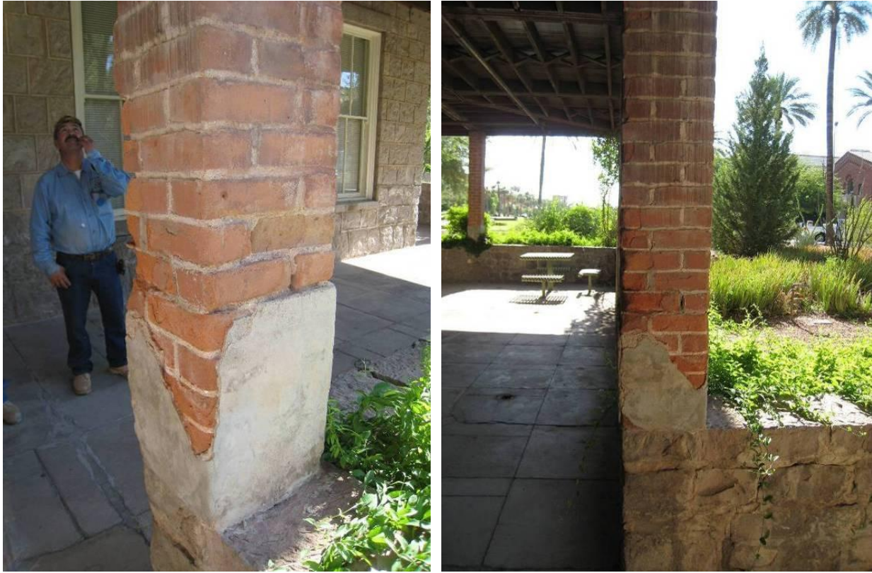
Figure 33- Pier #50 at SE corner of porch. The brick has been seriously eroded by the action of water and salts.
