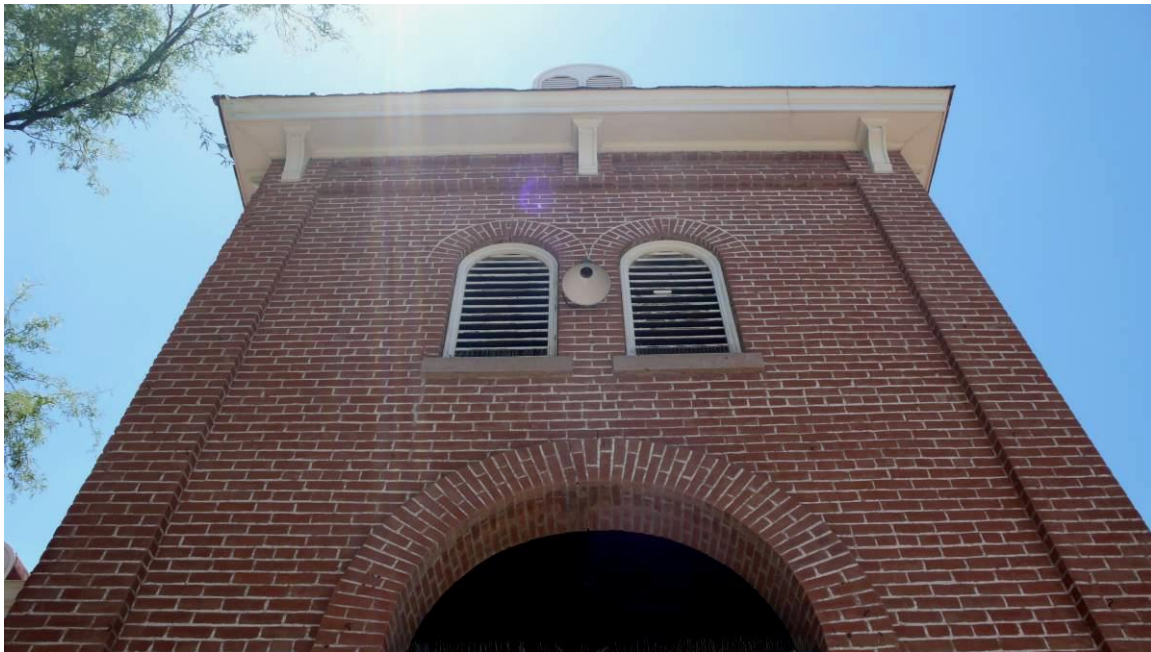
Figure 42 - East wall of east tower: cracks at key-stones of arches at entry towers, east & west. These will require re-pointing
