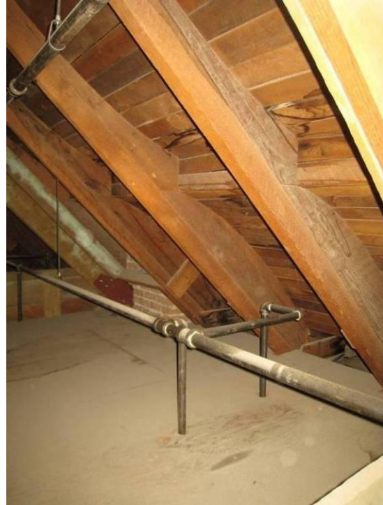
Figure 22 - Convex lower curve at Mansard framing; note fire sprinkler piping and plywood floor at attic.
