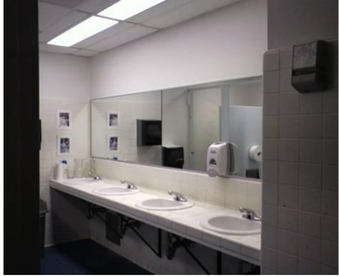
Figure 65 – Second floor restroom first approach presents an aged tiled counter supported with steel brackets.
