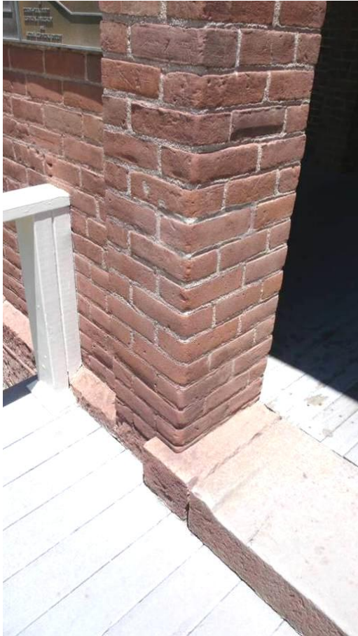
Figure 44 - Worn brick and threshold stone at west tower.
