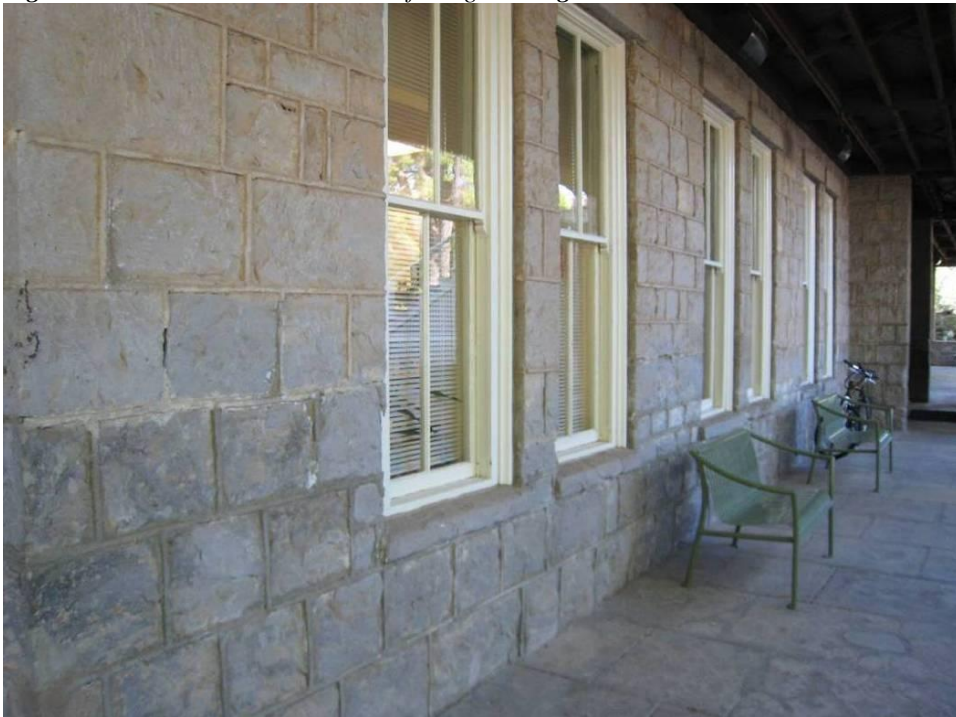
Figure 51 - East wall of first floor displays discoloration to height of rising damp in stone.
