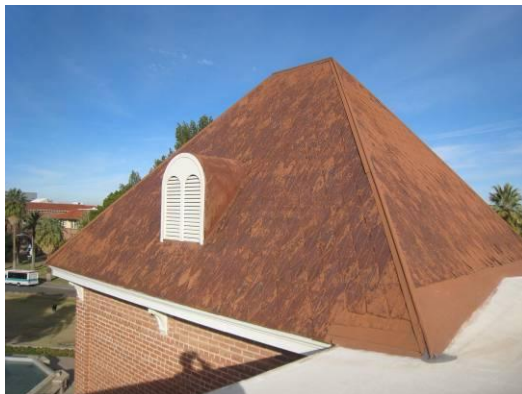
Figure 4 - Areas of rust and painted repairs at pyramidal roof of west tower.
