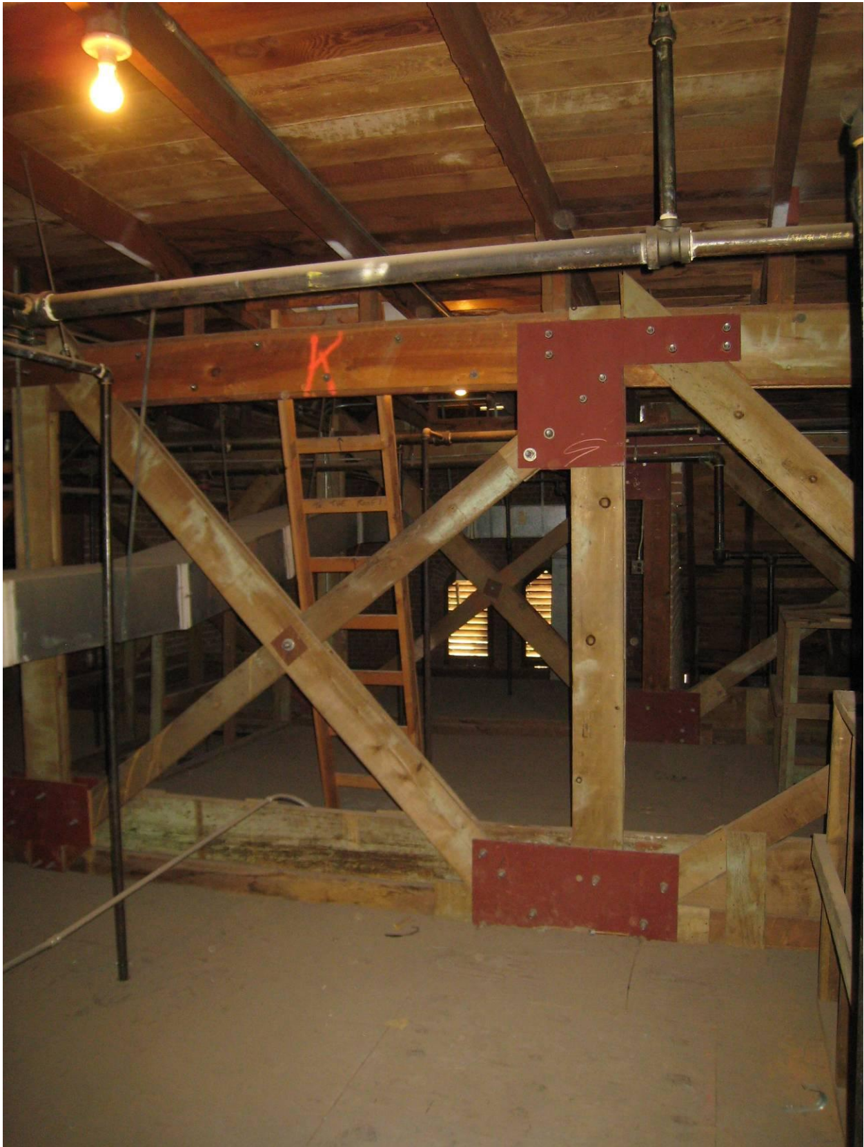
Figure 20 - View of typical truss at center section; note secondary roof joists propped from top chord for slope, and numerous repairs made to trusses over time. Despite apparently haphazard nature of repairs, structure is well tied together and presently stable. Duct at left of photo runs to east tower ceiling for air intake.
