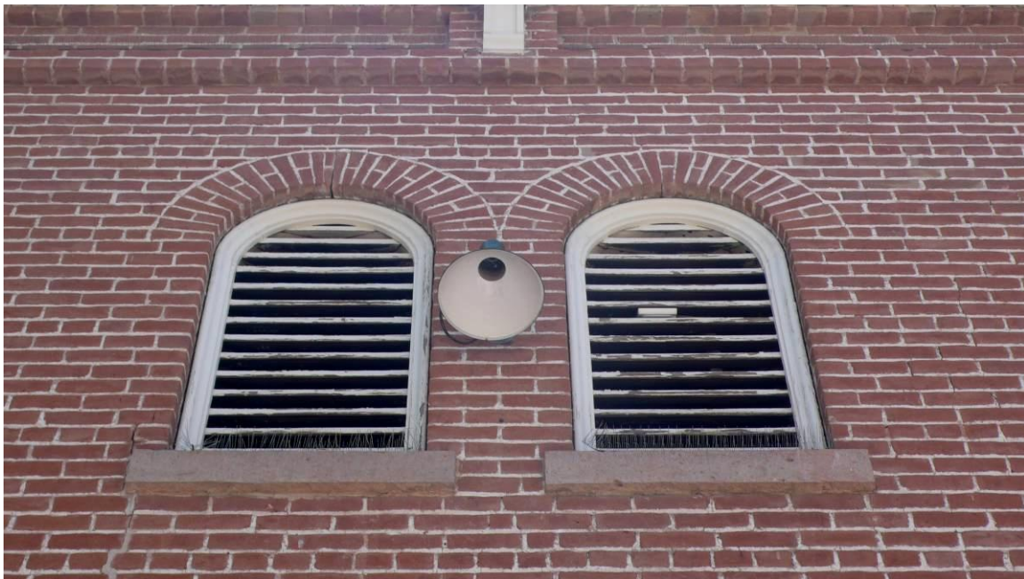
Figure 43 - Shear cracks through brick at left side of sill of left-hand arch at east tower should be monitored.
