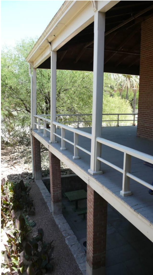
Figure 40 - Porch piers & posts significantly out of plumb; piers #5 & #6 at NE corner of east wing.
