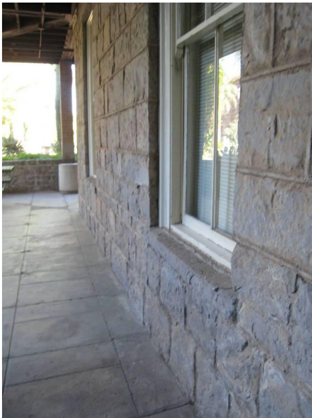
Figure 46 - The level to which moisture rises is evident in the discoloration of stone in the lower section of the wall, up to and above the sill level. Two-thirds of the sills at the 1st floor (40 out of 60 ) are deteriorated through salt erosion and must be replaced .
