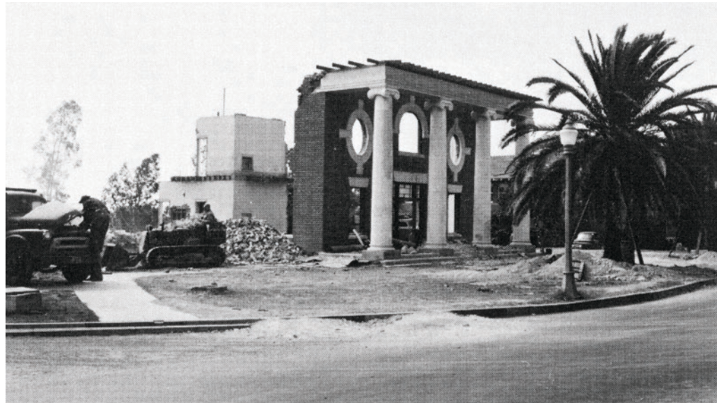
The 1958 destruction of South Hall, a dormitory building designed by prominent southwestern architect Henry Trost and constructed in 1899.
